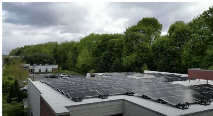
The law firm of Selingo Guagliardo, LLC has replaced the original solar panels on its Market Street building with 134 dual-sided solar panels that collect energy from both sides.
